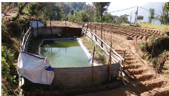
Plastic Pond constructed for rain water harvesting as part of Eco-village program
