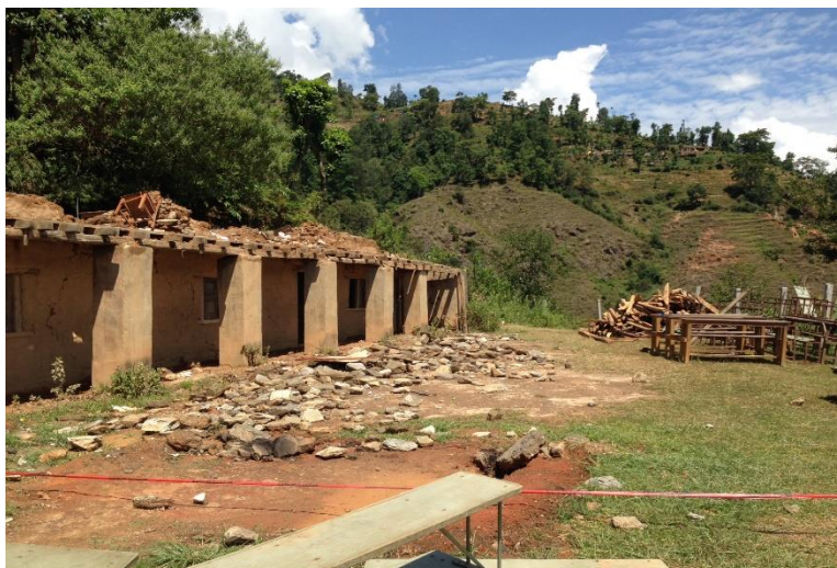
Damaged classrooms of Shree Panchakanya Prathamik Vidyalaya, Melamchi – 1, Sindhupalchowk
